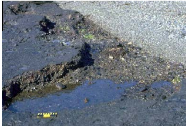
Figure 83: Asphalt Pavement (Cohesive, Heavily Oiled Surface Sediments)
