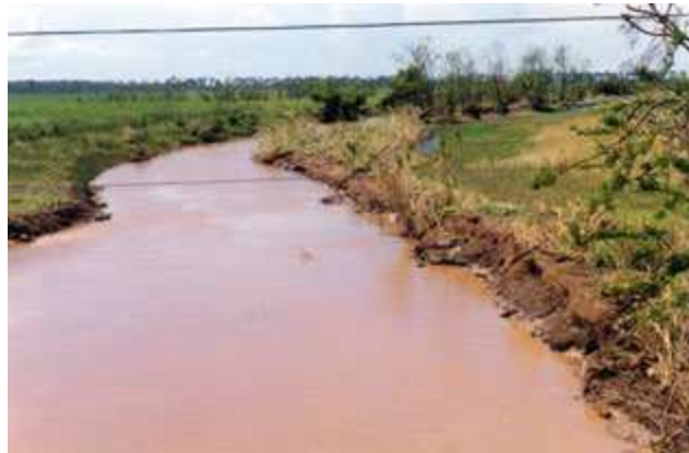
Figure 50: Exposed Scarps and Steep Slopes in Clay
